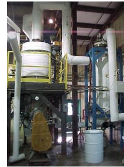
Hazen Research Facility FBSR Pilot Plant #2 of 5
