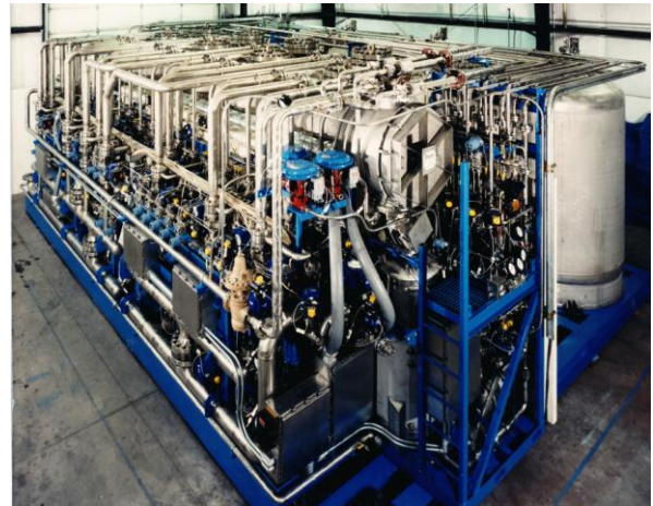
Modular Ion Exchange System, 9 inch steel shielding, 1500 gpm, full remote operation including backwash filtration system
